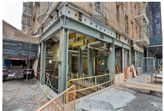
Entrance 1 (southeast corner of 63rd Street and 3rd Avenue) structural steel work
